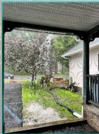
During a torrential downpour, rain was even coming out of the gutters.
